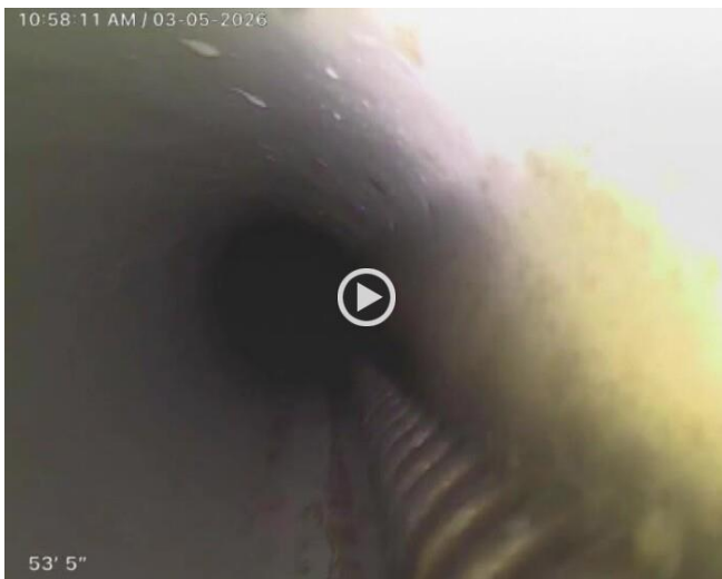
After Clearing Stoppage/ Calcium Build Up
